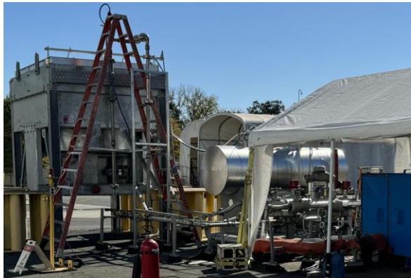
500kW demonstrator used to successfully heat compressed air and thermal oil
